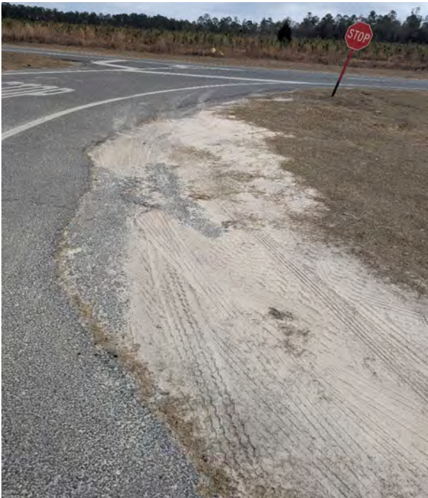
VISIBLE RUTTING FOR EASTBOUND RIGHT
