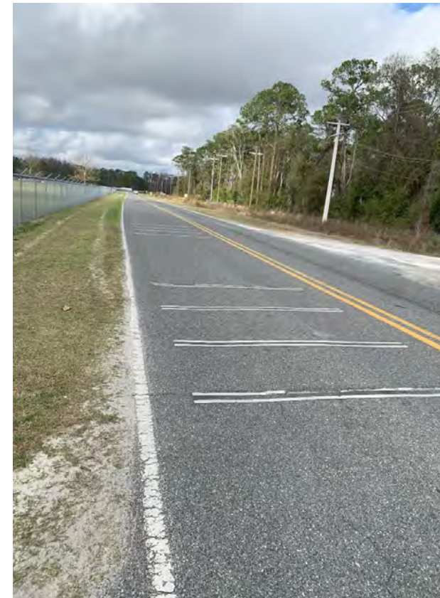
WORN RUMBLE STRIPS ON EB APPROACH
