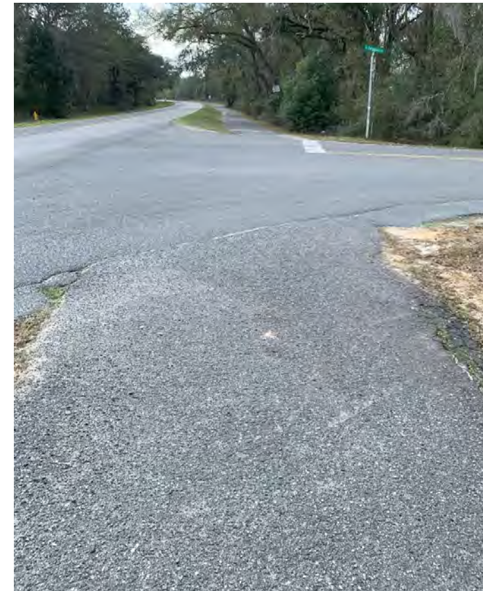
NO MARKINGS FOR SHARED USE PATH
