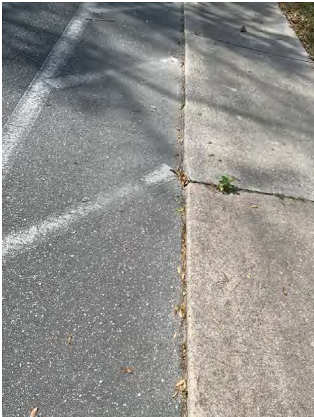
SIDEWALK IS FLUSH WITH ROADWAY AT TIMES
