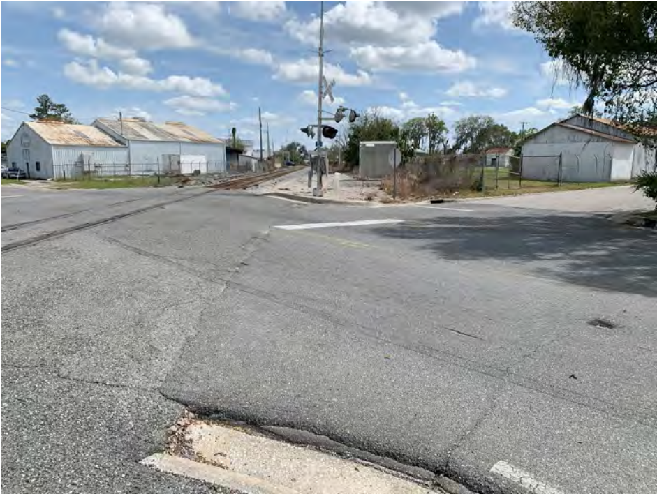
AWKWARD INTERSECTION APPROACHES AT RAILROAD CROSSING
