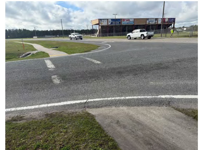
WORN CROSSWALK MARKINGS ON WB APPROACH
