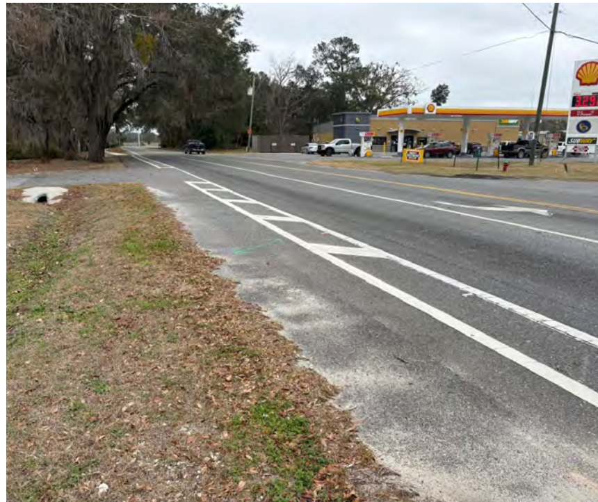
MISSING SECTION OF SIDEWALK
